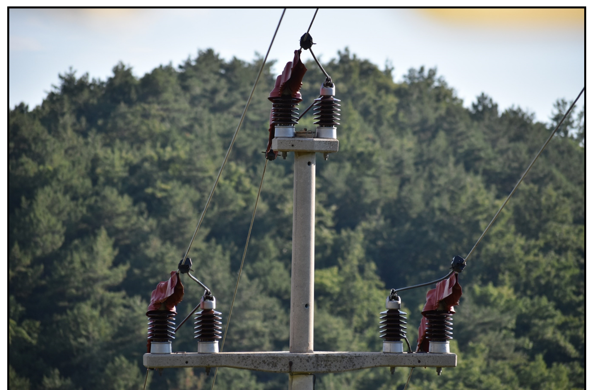
Mitigated middle voltage powerline pylon within the SPA „Kras“ (photo: P. Höfferle)
